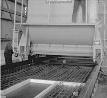
Figure 22: Concrete is discharged at a controlled rate by an electrically operated concrete spreader
